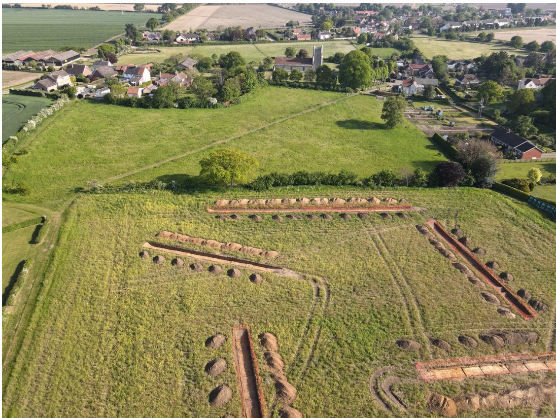
These substation survey works are very close to the village of Friston and actually encroach on some resident's back gardens
